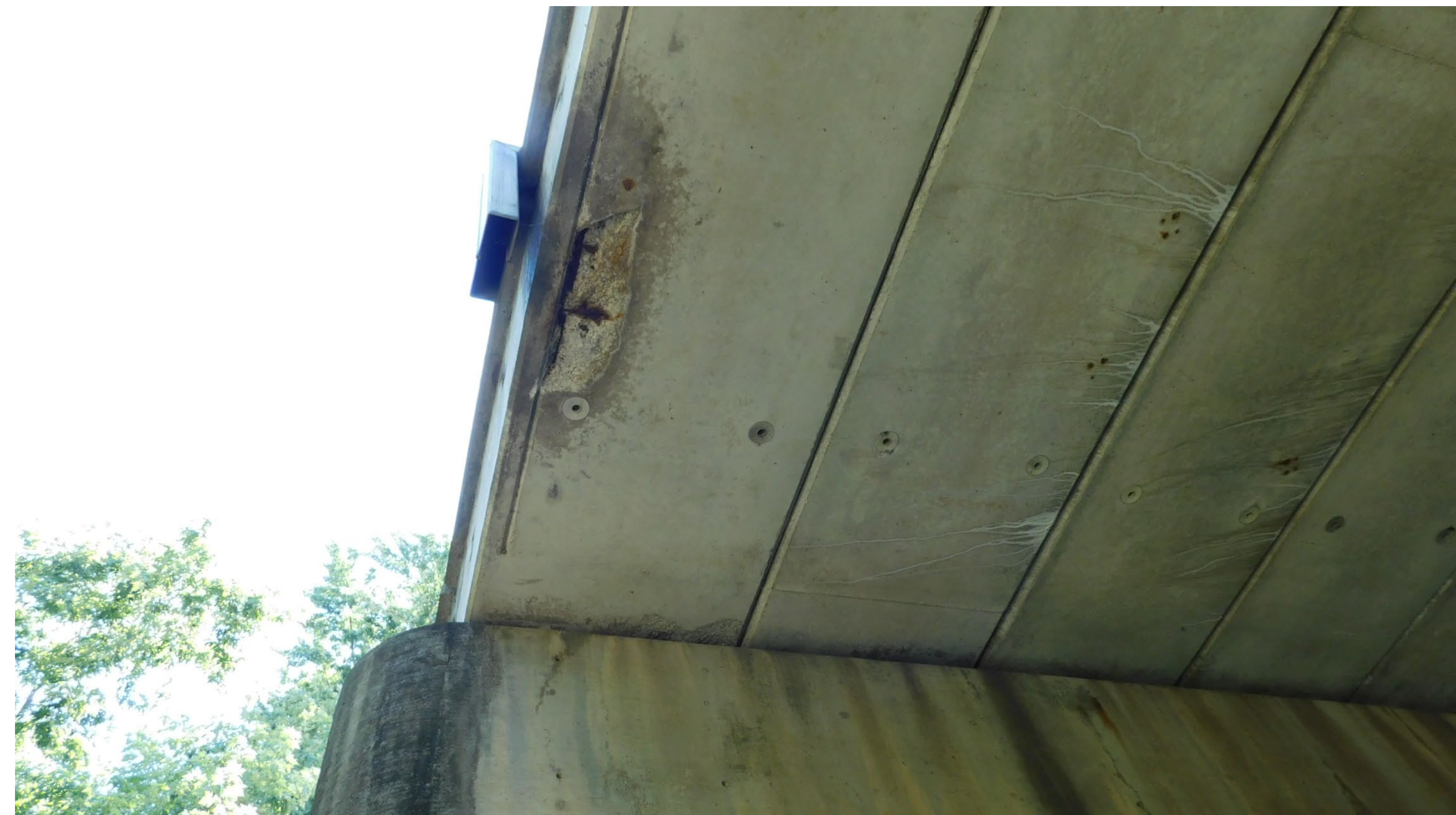
Exposed rebar at underside of beams
